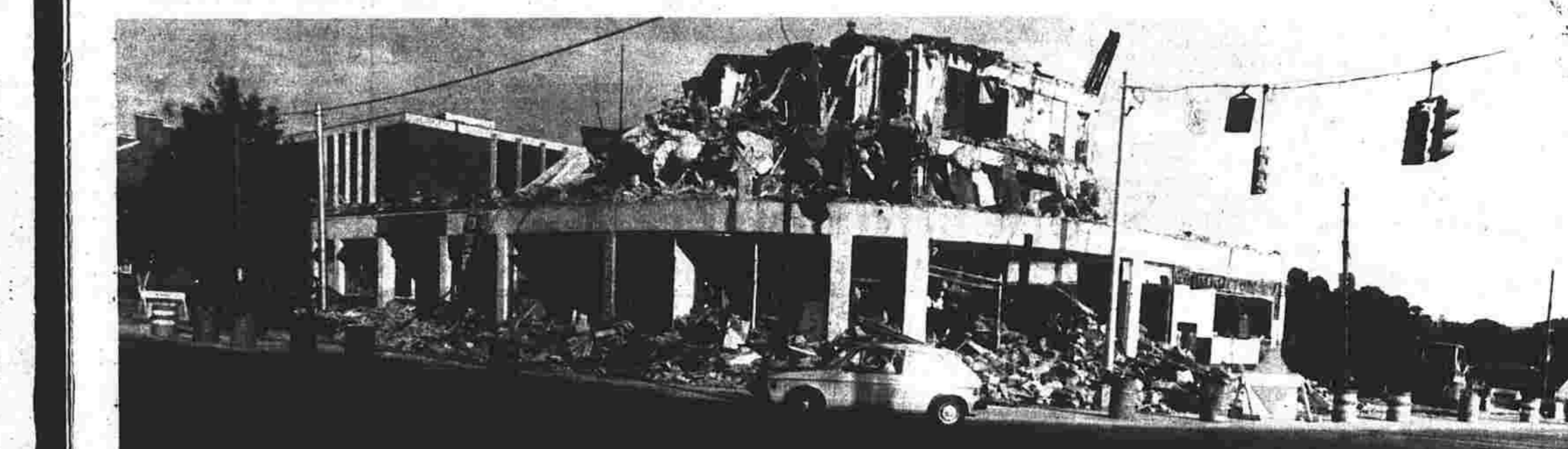
THIS IS HOW THE ODD FELLOWS BUILDING LOOKED FRIDAY EVENING, AFTER THE WRECKERS HAD BEEN WORKING IT OVER. The sturdy building was extremely hard to knock down. But it had become an eyesore.
